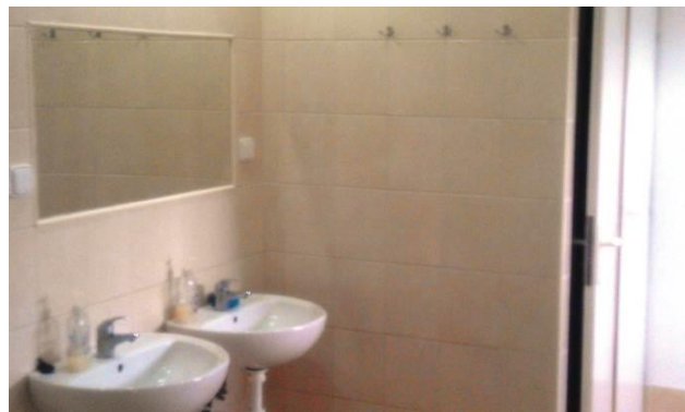
Picture No.8 Sanitary equipment
